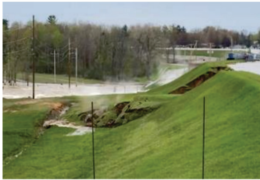
Embankment Instability Failure
